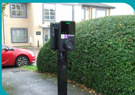
New Wetherby EV chargers
