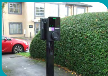
New Wetherby EV chargers
