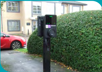
New Wetherby EV chargers
